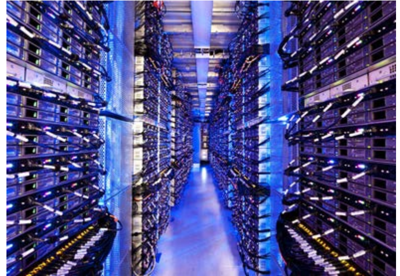
The Data Center
