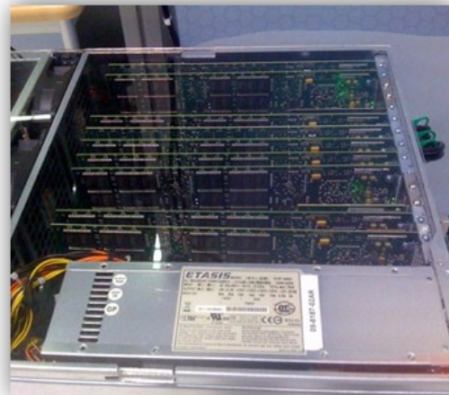
Data Center SSD Storage Array
