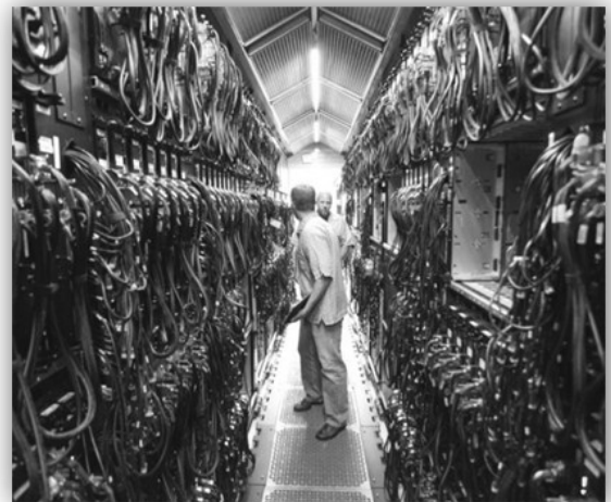
Data Center HDD Storage Farm
