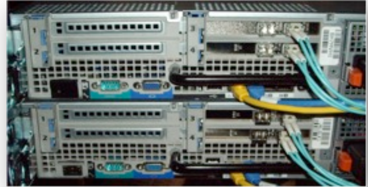
10GbE Server Connections
