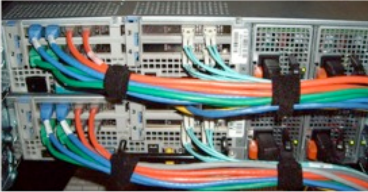
GbE Server Connections
