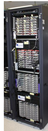
Flash Hammer Rack of 96 SATA Drives
