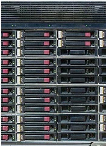
Legacy Storage Array
