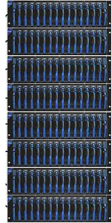
Dense Server Rack
