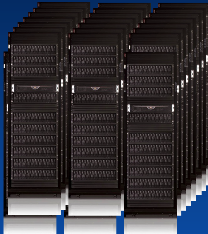
Major Storage Vendor 37.6 racks
